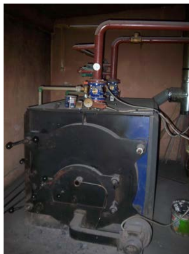
Boiler Project for Onesimus Home for Boys
